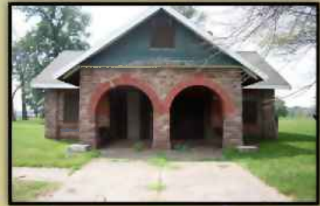
The range house, the only structure remaining from the once nationally recognized Bay View Range, has fallen into disrepair and is in need of restoration.
